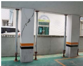
Fig. 1 Failure of a shear-critical column
