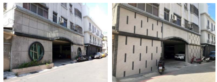
Before retrofitting After retrofitting Fig.2 Residential building in Hualien involved in the Interim Seismic Retrofit project
